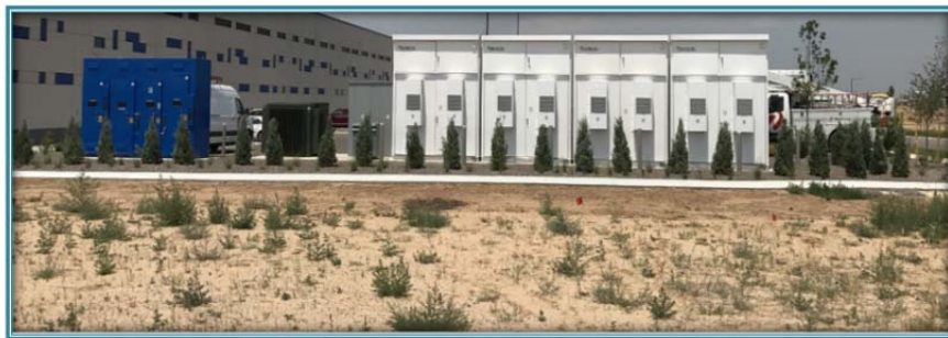
Figure 11: 1 MW Battery System
