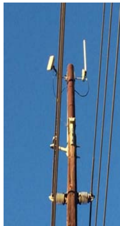
Figure 1: WiMAX portion of the FAN on a distribution pole
