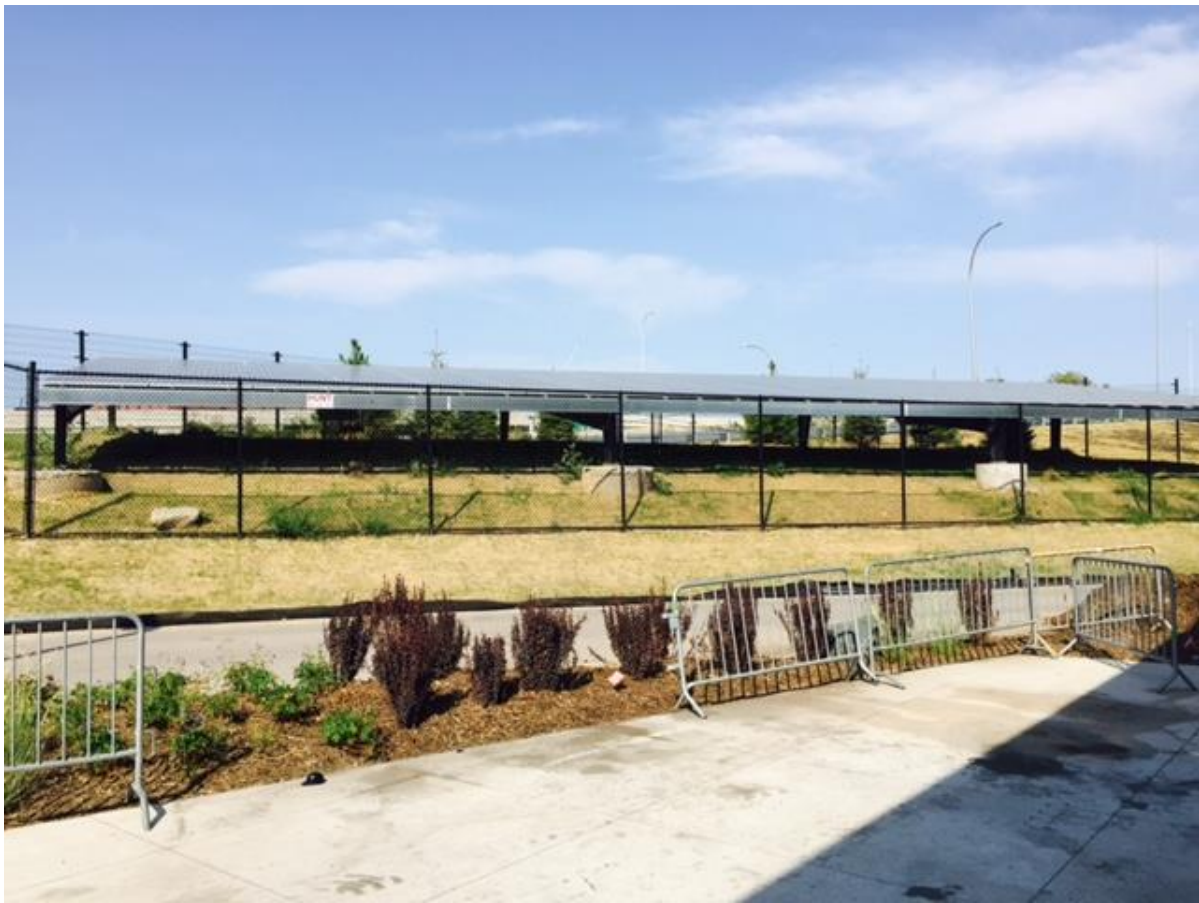
Image 10. Completed northeast solar array; September 9, 2015
