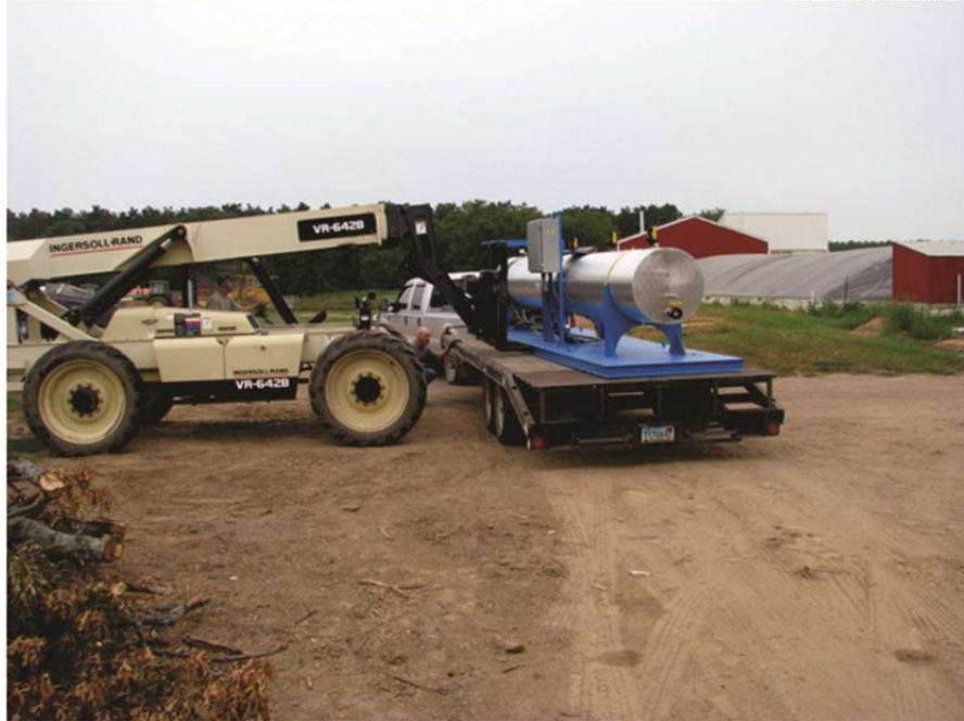
Figure 32. Photograph of pilot-scale anaerobic digester vessel during installation. The full-scale digester is visible in the background.
